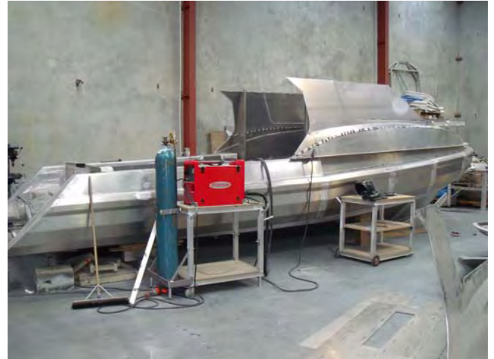
New build – with welding deficiencies.
